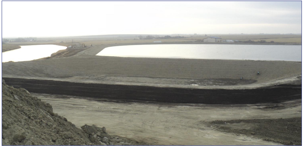
Construction of the new Rocky View water treatment plant looking south east toward the treatment plant from the north west end of the Stilling Basin. Graham Creek Reservoir can be seen in relation to the new construction. Photo submitted by MPE Engineering Laurie Manion
