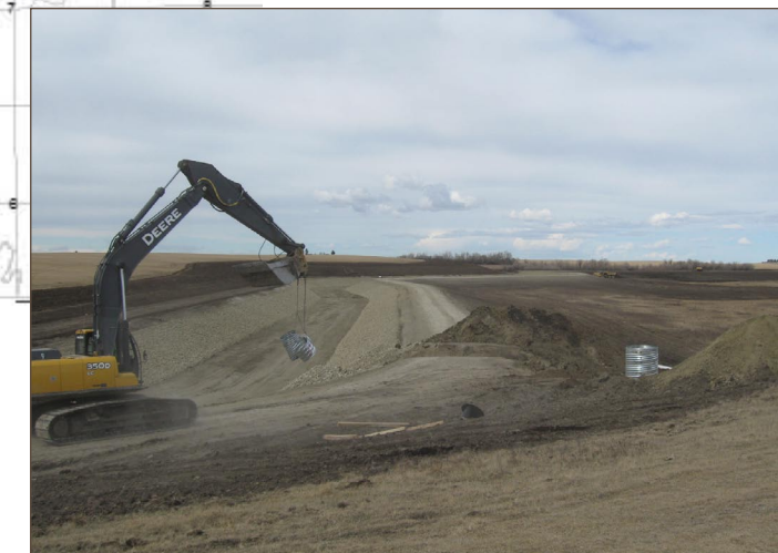
This is the same section of A Canal at the end of rehabilitation. Putting in a turnout. WID photo
