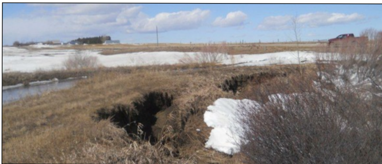
Flood Damage Along North A Canal - WID Photo
