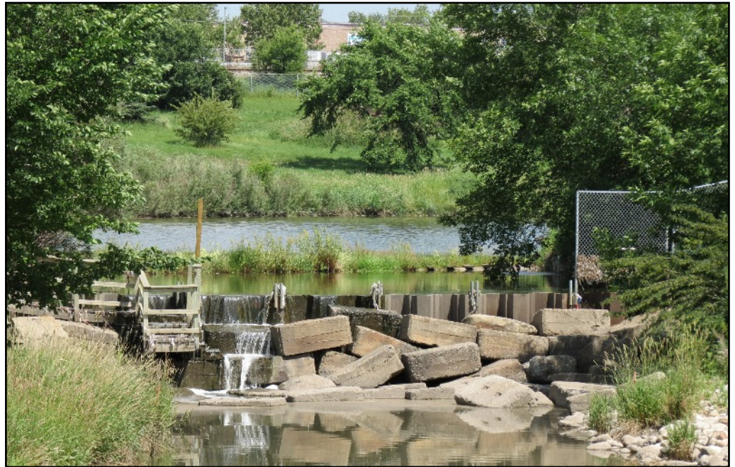
Storm Water Pond "Duck Pond" at 61 Avenue in Calgary - Kristi Cox - photo
