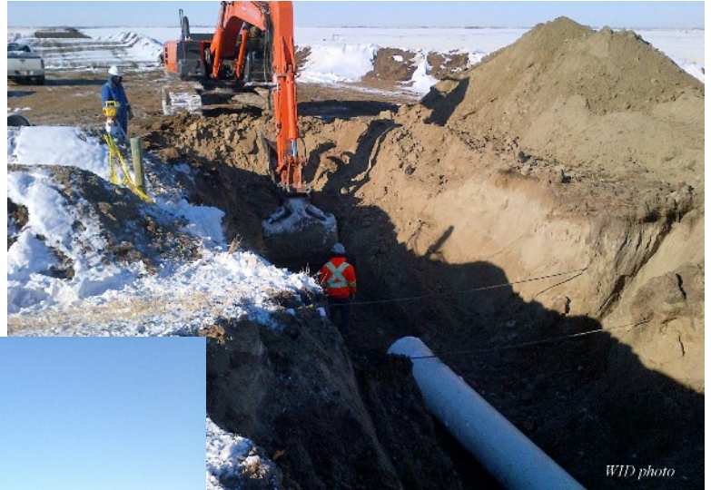
The Sheep Camp pipeline ties to the pump station installed last winter
