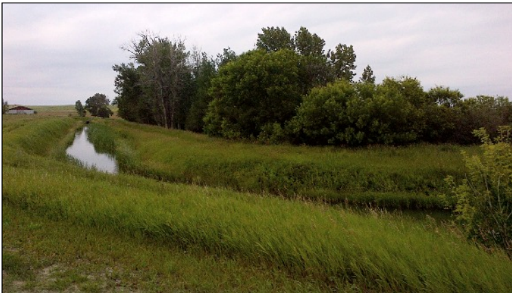
Before rehabilitation, canals lose water to seepage and plant growth and banks are prone to erosion. Top photo shows after rehabilitation at the same location - WID photo
