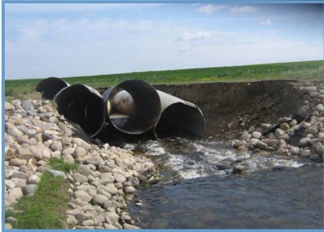
Major crossing failure on the "B" canal
