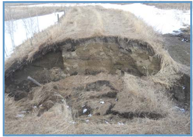
Complete bank failure on a main supply canal
