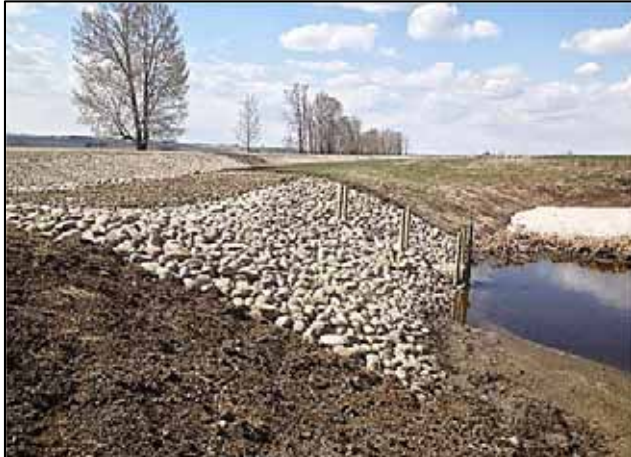
Spring washout repair east of Strathmore
