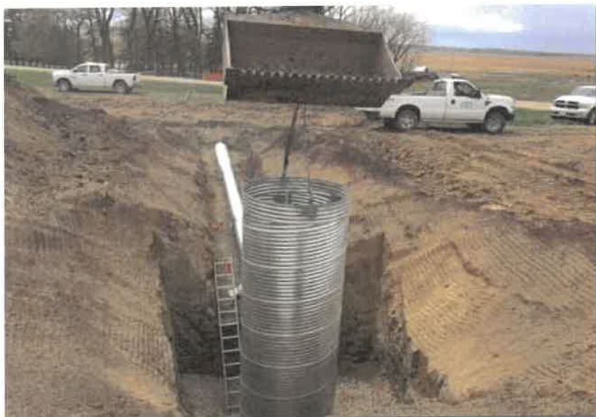
Irrigation standpipe and inlet installation for turbine pump application
