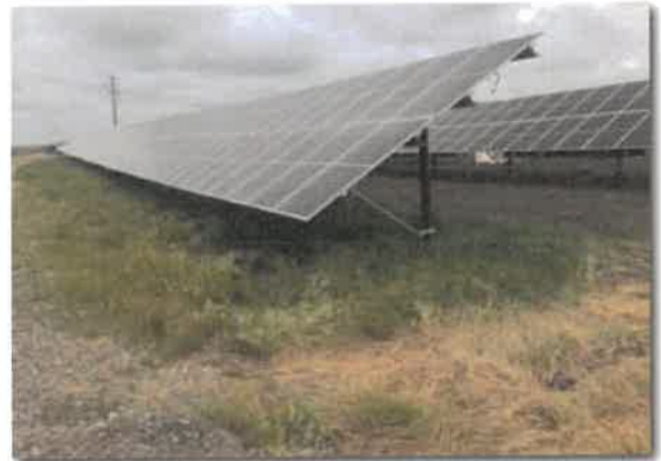
Solar generation system
