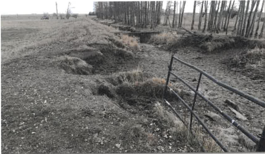
Ditch rehabilitation and fencing required on old ditch south of Strathmore; fenced dugout storage and offsite watering systems prevent this type of damage
