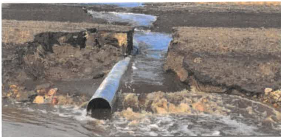
Spring runoff 2019 washed out culvert
