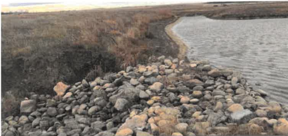
Erosion repair required on irrigation pump site reservoir
