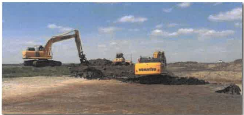
Major storage upgrade for irrigation pumping
