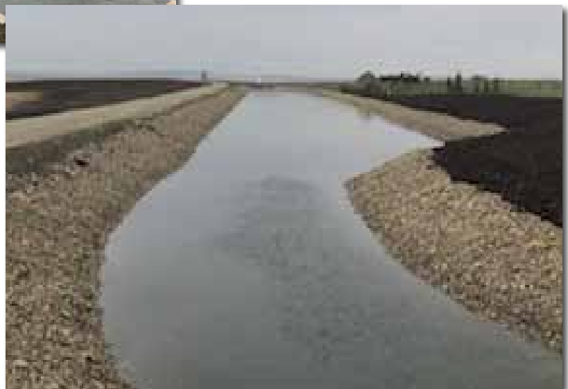
Extra wide right-of-way incorporated into canal design
