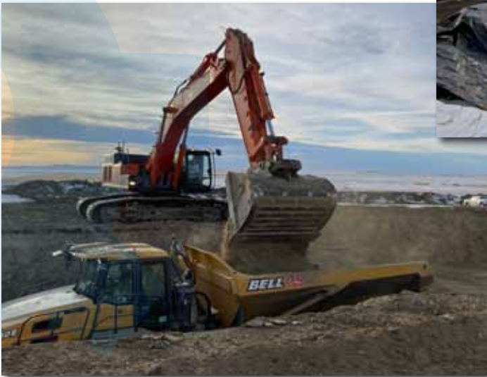
Clay loaded from borrow pit within WID lands for compacted liner cover
